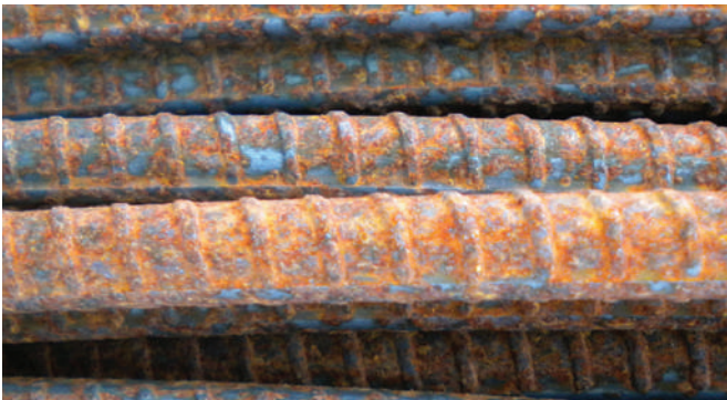
Figure 5 – Close-up view of the #3 bars showing a tightly adhered rust pack and good deformation definitions.
